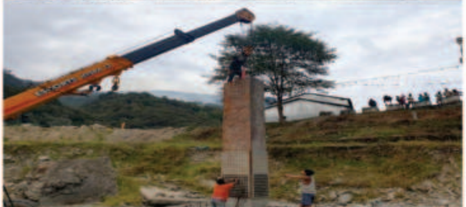
Steel Composite Bridge over River Tawangchu on Lhou Nallah to Mukto Road (Span-80m) in Tawang District of Arunachal Pradesh under CRF
