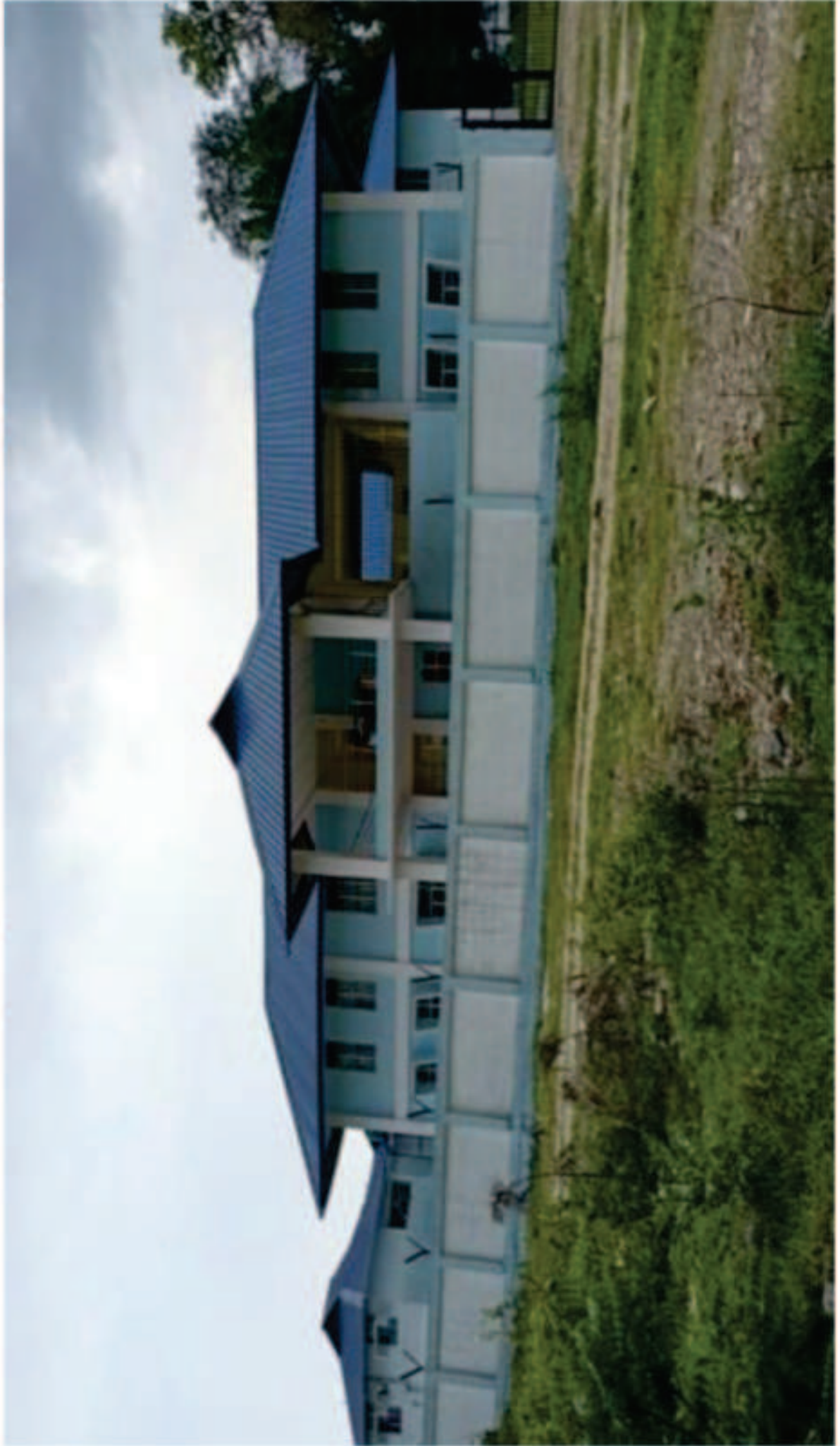
Creation and development of premanent structure for hostel block ANM nursing school, Pasighat.
