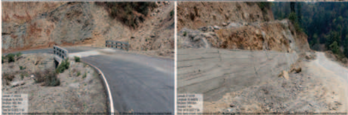
Name of Work:- Improvement of Road from 9 mile point of Bomdila-Tawang road to Salari-Nafra Road (36.00km) in West Kameng District (Phase-I) km 0.00 to 20.00 km under EI Schemes in the state of Arunachal Pradesh.
