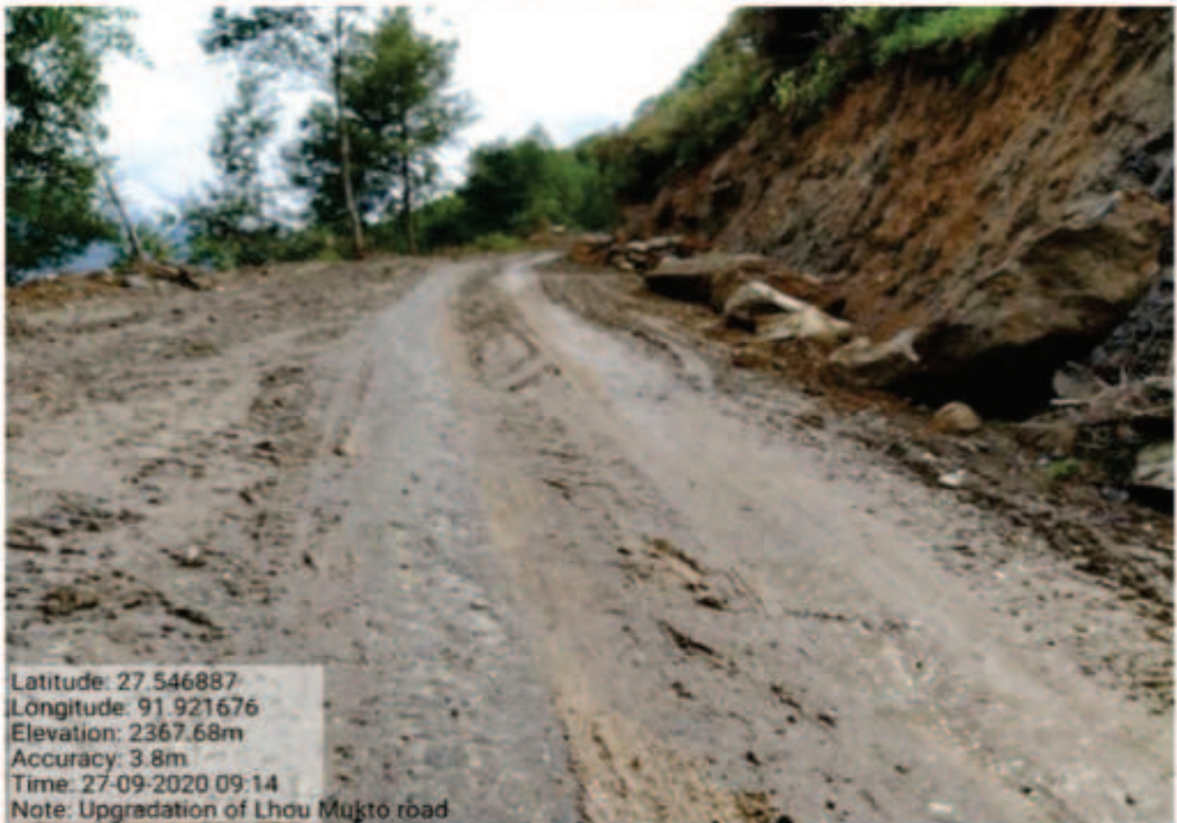
Upgradation of Lhou- Mukto Road to Double Lane Specification (12.50 Km) Under CRF Scheme in the State of Arunachal Pradesh. Under CRF
